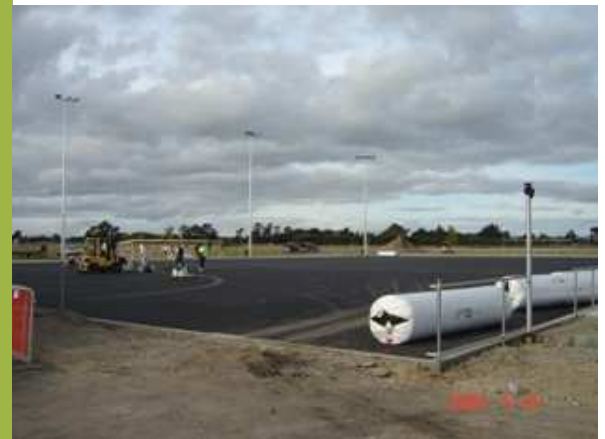
The turf just about to be laid and the new dugouts going up in the background
